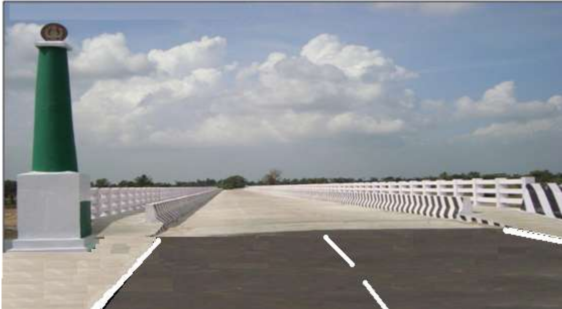
River Bridge on Kazhiyur-Athi Road across Cheyyar River opened on 27.01.12 by the Hon'ble Chief Minister
